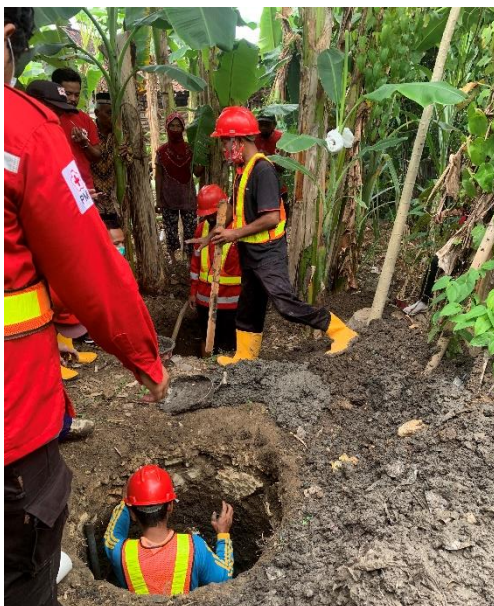
Use of PPE on Training of Septictank Construction for Volunteers of the Indonesian Red Cross (Palang Merah Indonesia/PMI) in Sragen District, Central Java.
