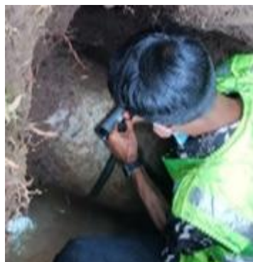
Staff of USAID-SECO Partnership demonstrating the installation of sensors of a leak noise correlator to staff of Perumda AM Kota Magelang
