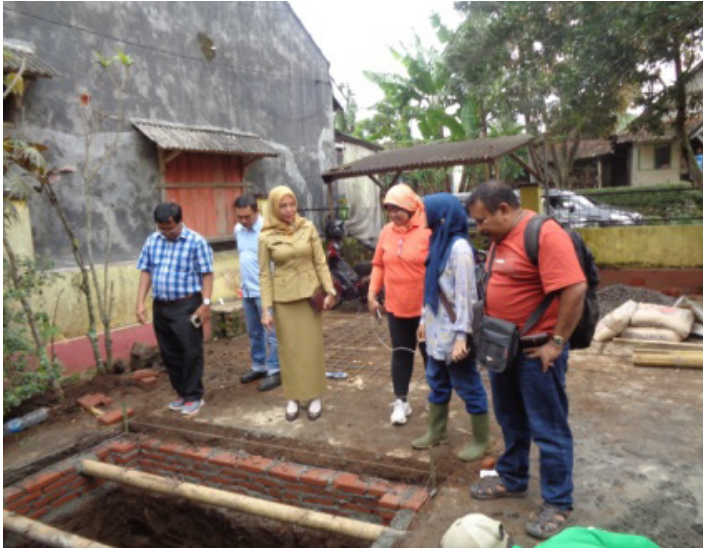
Field monitoring on the construction of infiltration ponds conducted by USAID IUWASH and CCFI in Ketindan Village, Lawang Sub-District of Malang District.
