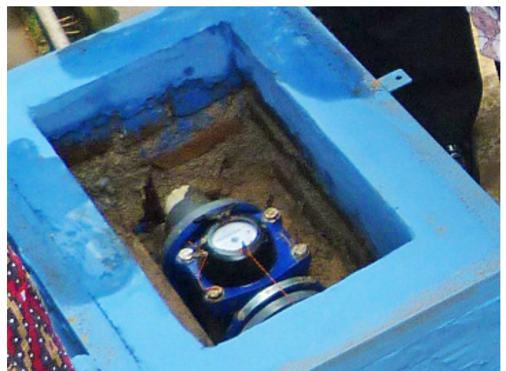
A newly installed Master Meter in Kapatang Village, Sibolga City of North Sumatra.
